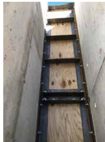
Fig. 6: A downstream view of an abutment used to provide a seal between the tank wall (left) and sides of the precast modules (right)
