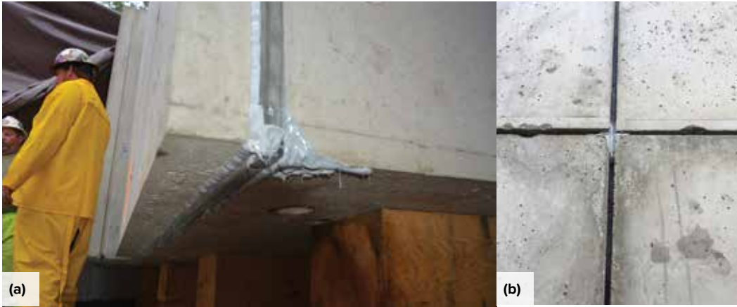
Fig. 5: Expansive waterstops were used to seal the joints between modules and between modules and the test tank base: (a) waterstops were installed in reveals in the modules immediately prior to assembly of the dam; and (b) as the modules were assembled, the waterstops were compressed against adjacent modules
